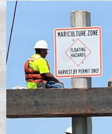
Photo by Dominic Guadagnoli/CRD A crew installs pilings and signage marking the Chatham County Shellfish Mariculture Zone on April 28. These pilings and signs will help notify boaters of potential hazards associated with floating aquaculture gear within the newly established commercial mariculture zone in Bull River just north of Pa Cooper Creek.
